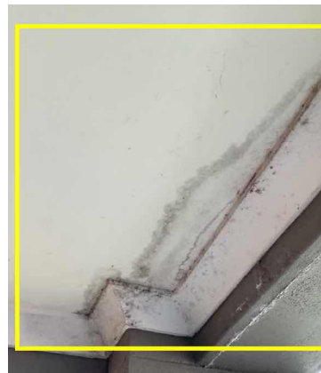
Clear evidence of leaks
